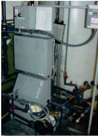
Figure 1: Ozone Treatment System
